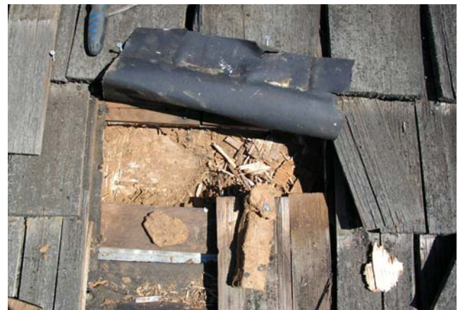
Existing roof exposed to deteriorated plywood over entry area
