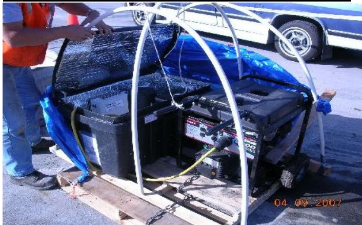
Geothermal Conductivity Test Equipment
