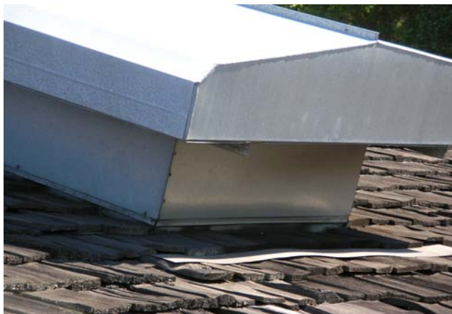
Existing ventilation unit
